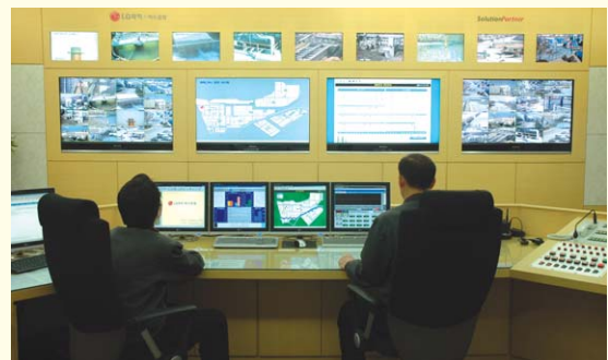
• Emergency Control Center at Yeosu Plant
